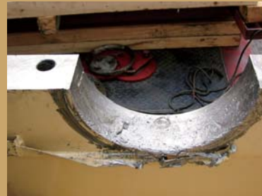
Fig 2. Damaged bearing housing to be repaired by metal spray
