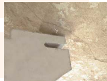
Hangerbeam status before test - right
