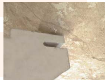
Hangerbeam status before test - right
